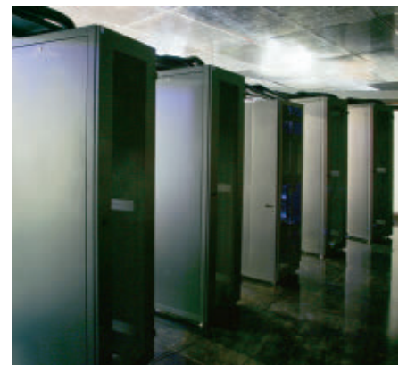
Texas server room
