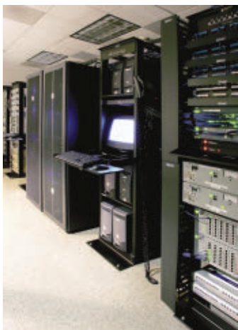
California server room
